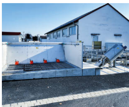
Sewer Sedimentation Reception Station – for collecting of sewers, gully waste and road sweepings
